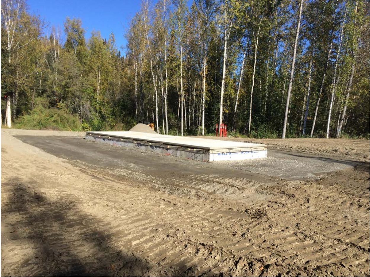
Figure 1 - Recently constructed thermal storage tank on the site.
